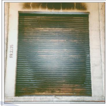
TACAM Shutter AFTER conclusion of 6 hours Fire Test. Fully intact; minimum distortion.
